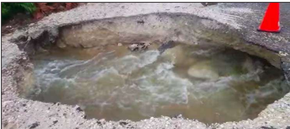
Road caves in on Philip Goldson Highway
