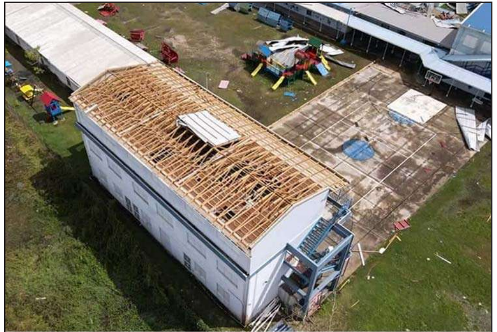
Belize Elementary School roof ripped off
