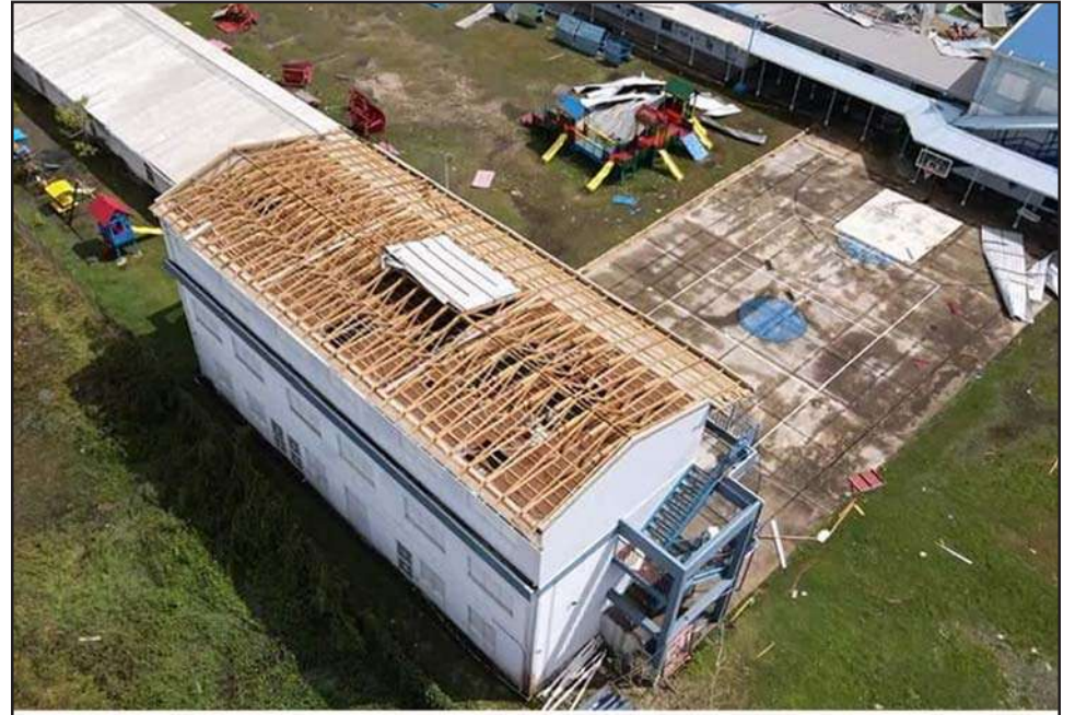
Belize Elementary School roof ripped off
