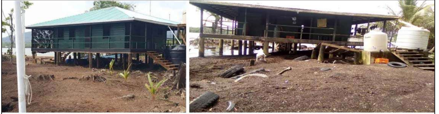
Sarstoon FOB at time of its opening vs Current condition
